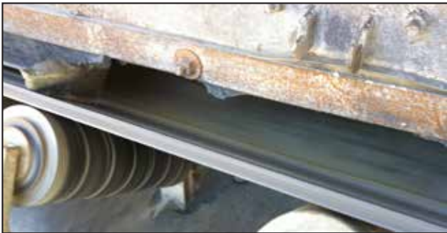
One of the most important jobs of the load point is to provide a seal that prevents material spillage and controls dust. In this photo, spillage and dust are likely because a proper seal is not attained.
