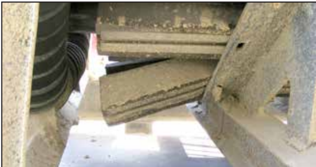
Knowing the material lump weight and drop height are essential to choosing proper impact point protection. If these numbers aren't taken into account, the impact bed will fail, as seen here.
