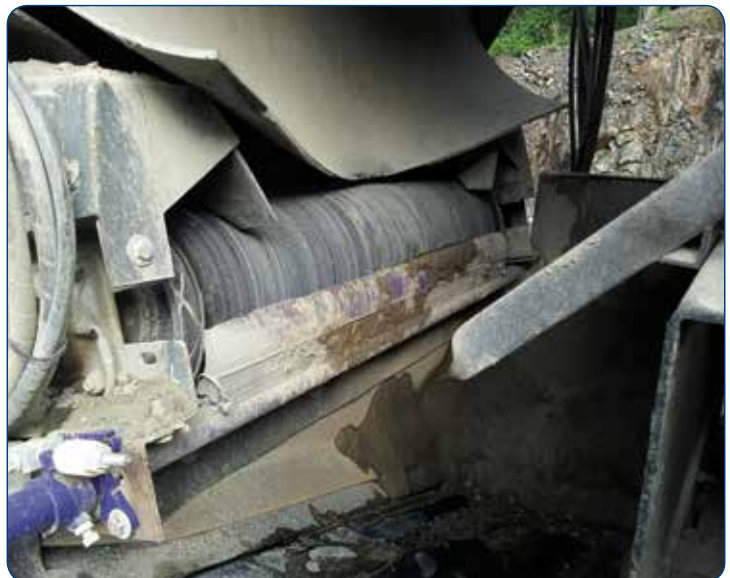
Rockline EZZ-LS fitted to conveyor at Woolgoolga Quarry
